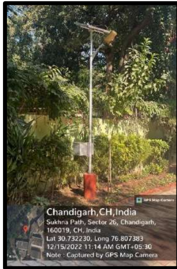
Solar Light in Boys Hostel
